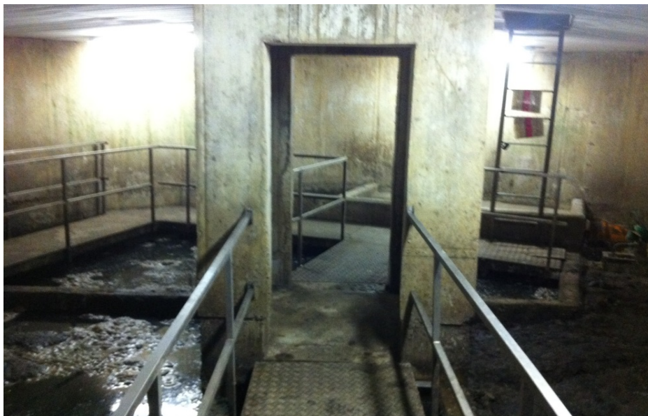
Figure 5: Inside the Sersjantvíkin WWTP at the 1st sampling round, in October 2013
